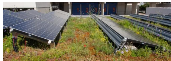
Figure 2: The two used mounting systems on the PV plant. On the left side the 20° tilted ZinCo mounting system for green roofs and on the right side the 15° tilted Hilti mounting system mostly used for flat roofs without greening.
