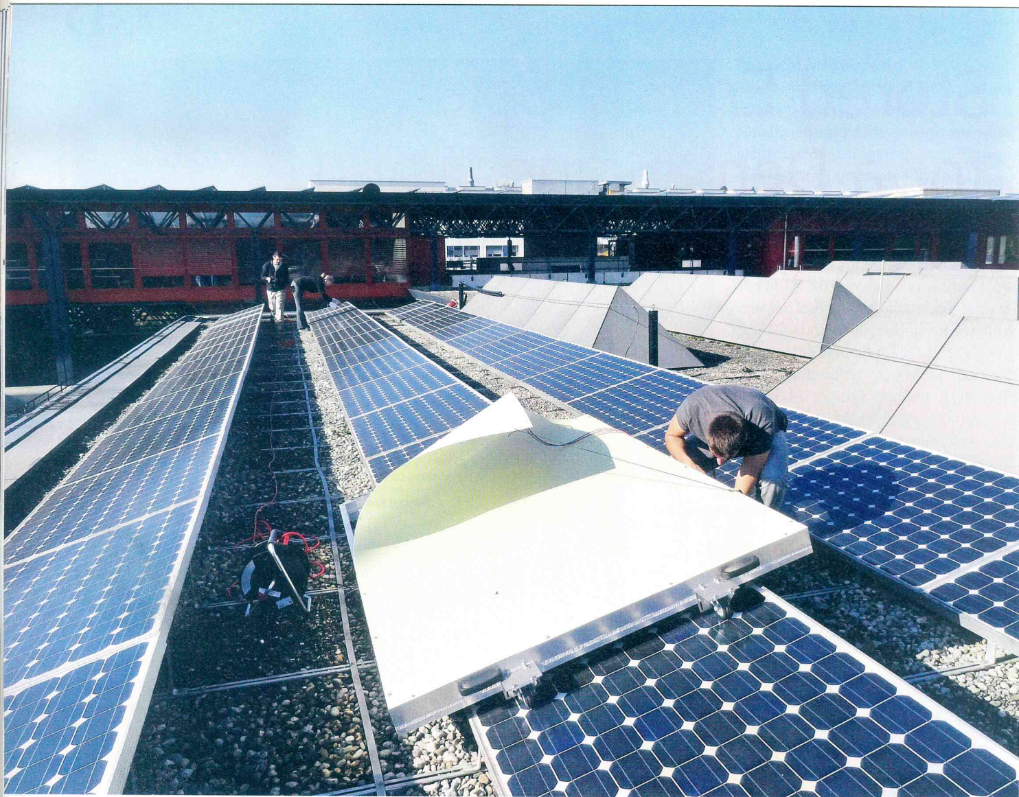
The mobile LED flasher, developed by Franz Baumgartner and Daniel Schär at the Zurich University of Applied Sciences, Switzerland, in action flashing a rooftop array.
